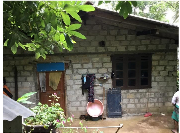
Figure 7b: Houses at risk of slope failure
